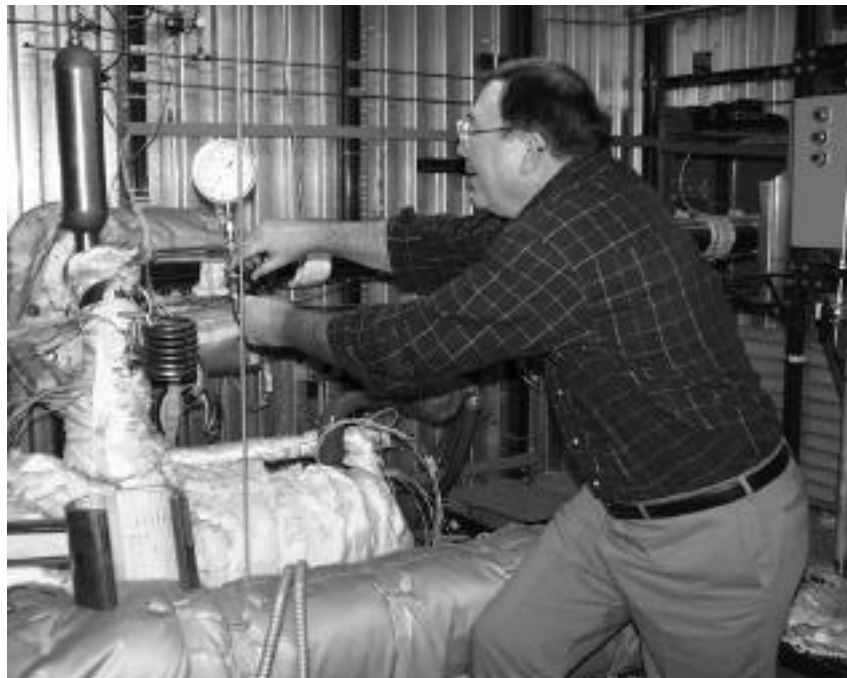
Figure III-2. An operating liquid-lithium pump system circulating 200 gallons/min (100 times the flow needed for the ISOL target) in the Argonne Technology Development Division.
